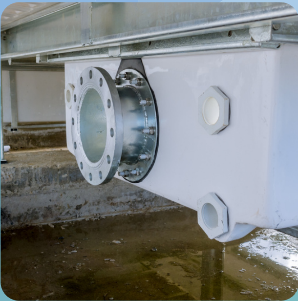
FRP. Water Sump
